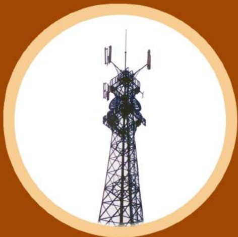
Communication Base Station
